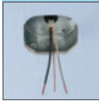
Ceiling box is set back from surface.
